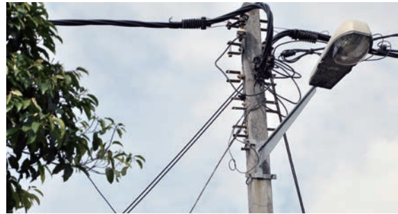
D-CCAP suspended installation in Malaysia
