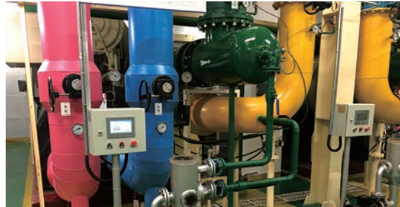
Cleaning devices for air-conditioning condensers
