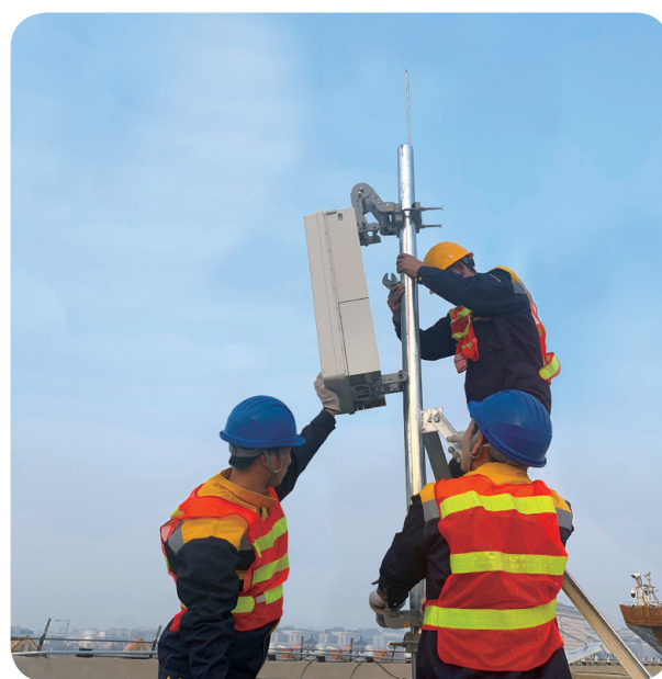
Installation of Huawei's 5G 64T64R AAU; Huawei's all-scenario 5G sites facilitate rapid, large-scale deployment of 5G worldwide
