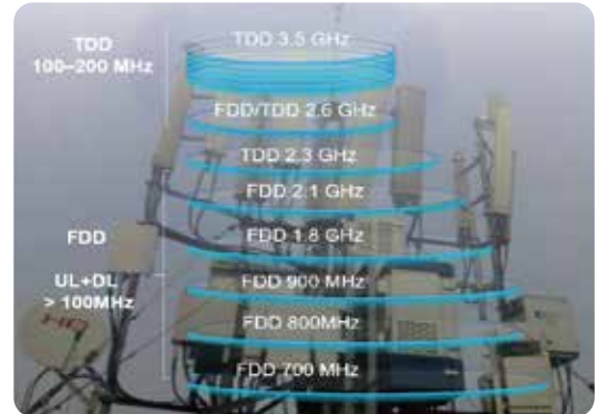
Figure 1 Multi-band deployment on a tower
