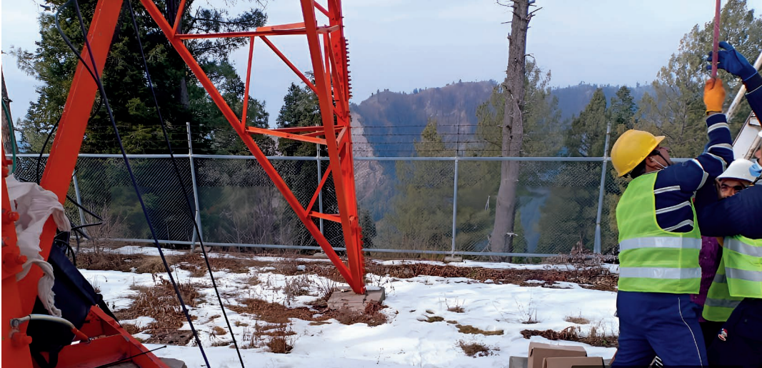
Field team busy at work, showing dedication while installing microwave dishes in extreme weather conditions
