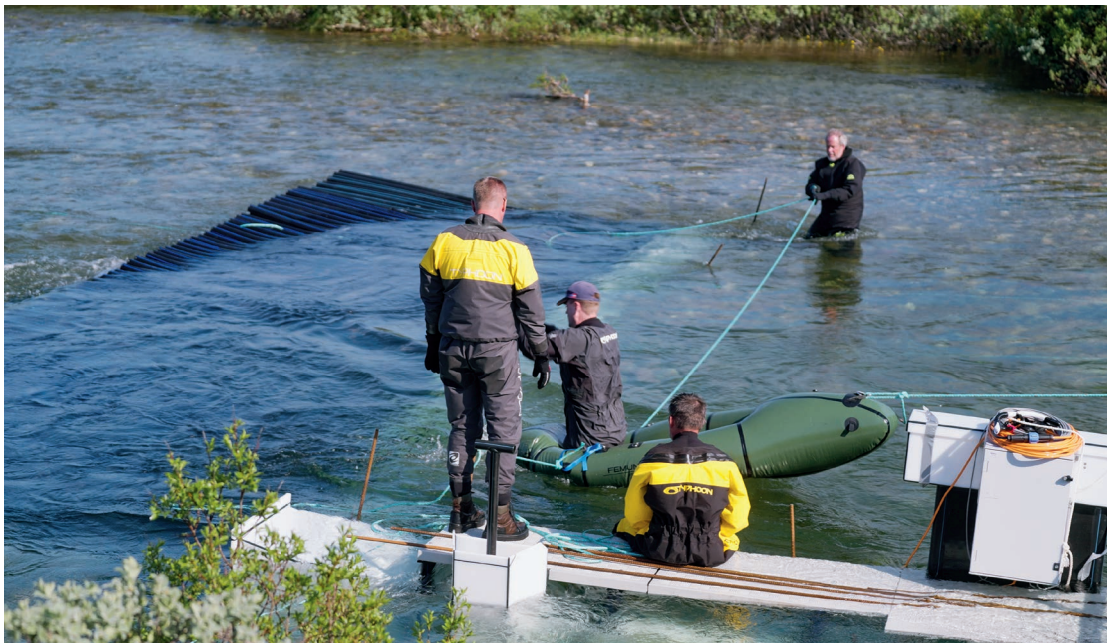
Working with volunteers to install the system (author standing on the left)
