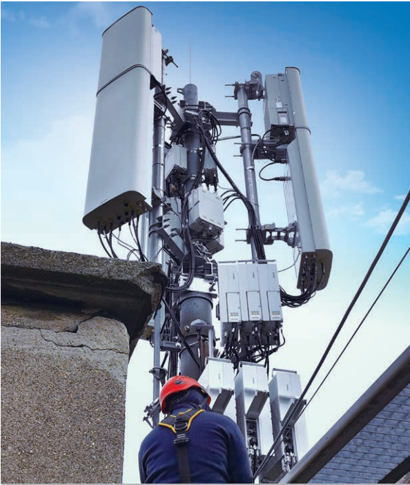
5G base station installation in Switzerland
