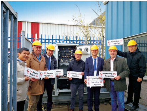
Customers visiting a site utilizing the 5G Power solution during the 2019 Global ICT Energy Efficiency Summit
