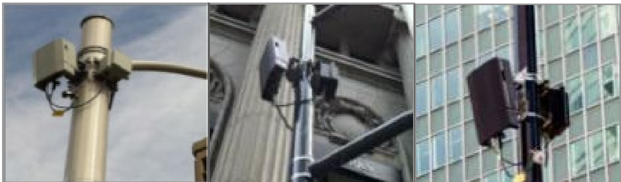
Figure 1-5 Deploying small cells on poles
