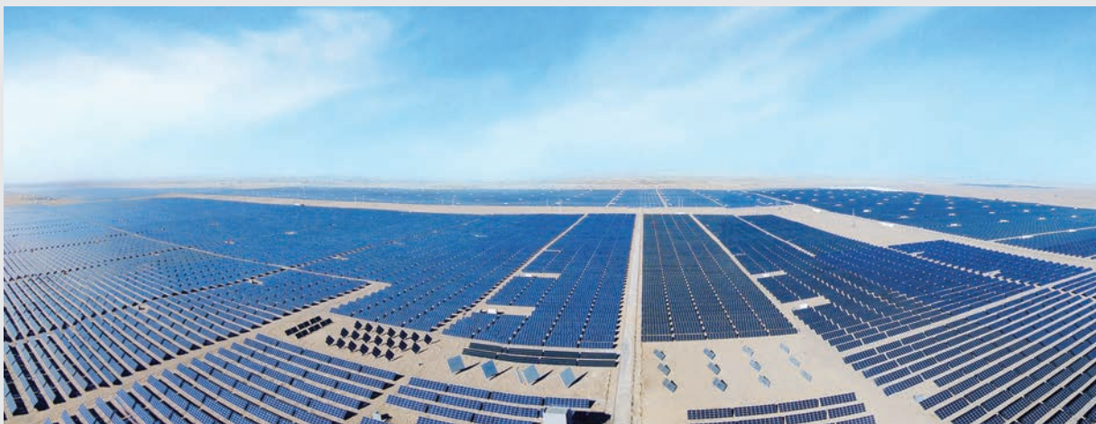
Digital and smart PV power station
